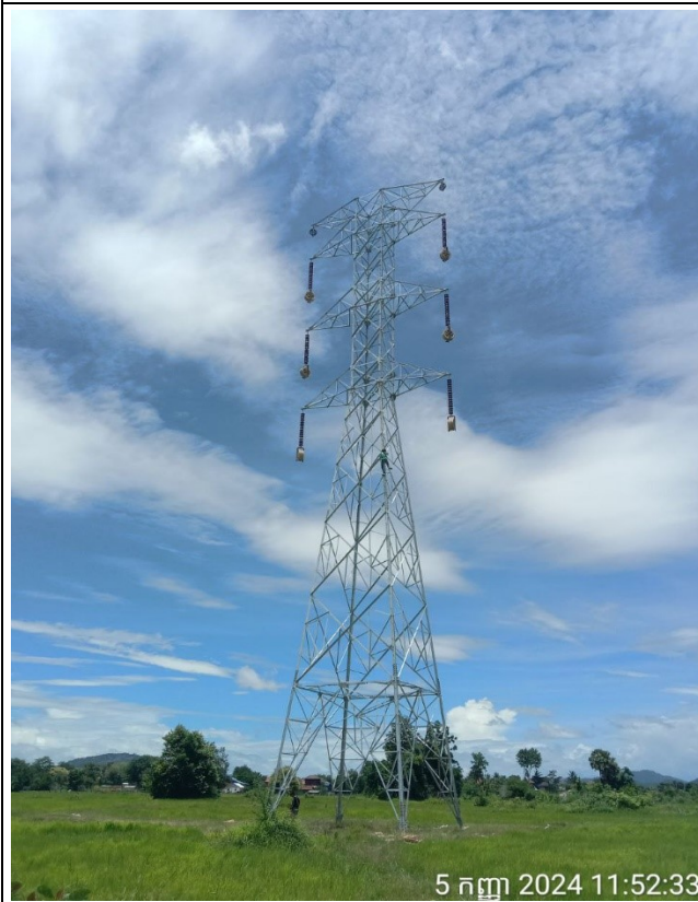
Hang insulator disk and roller.
