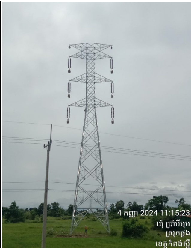
Hang insulator disk and roller.
