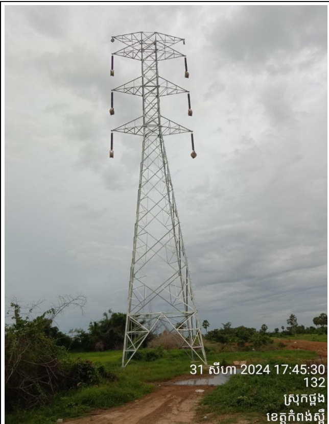
Hang insulator disk and roller.
