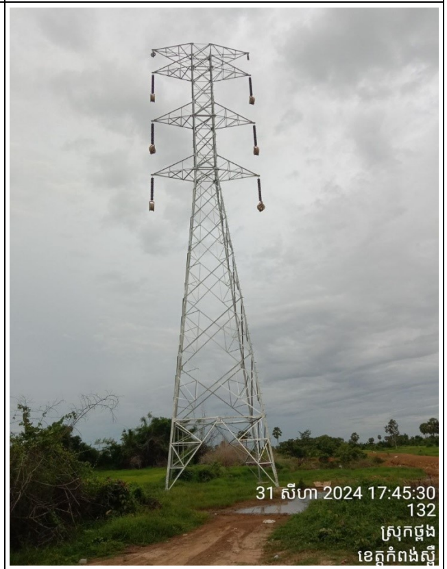
Hang insulator disk and roller.
