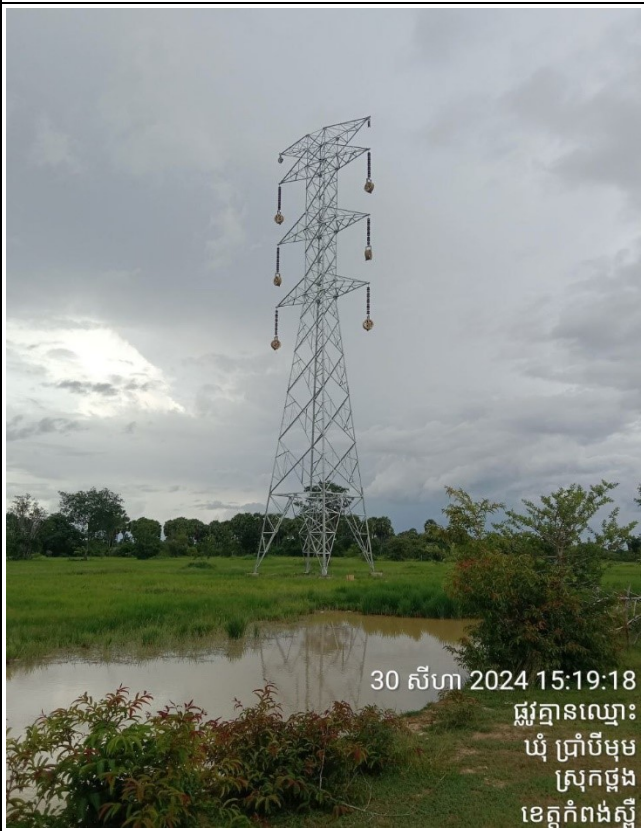
Hang insulator disk and roller.
