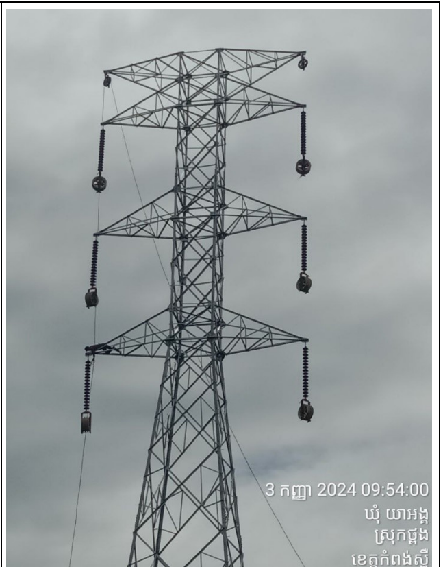
Hang insulator disk and roller.
