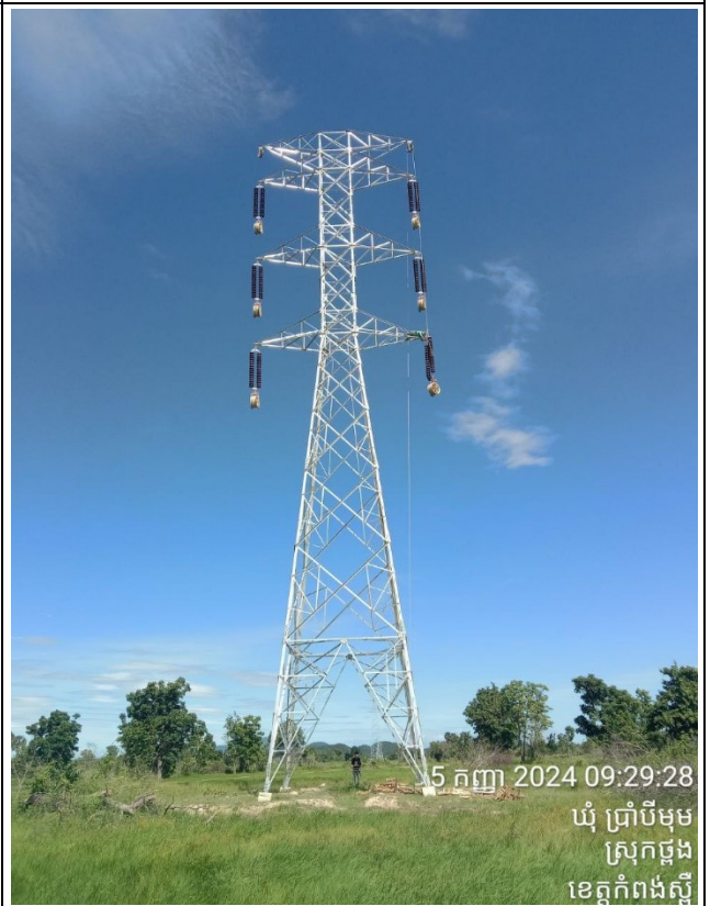
Hang insulator disk and roller.
