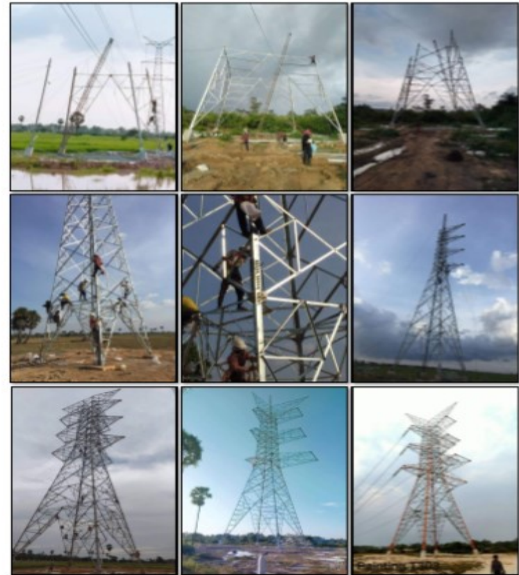
Structure of Transmission Line
