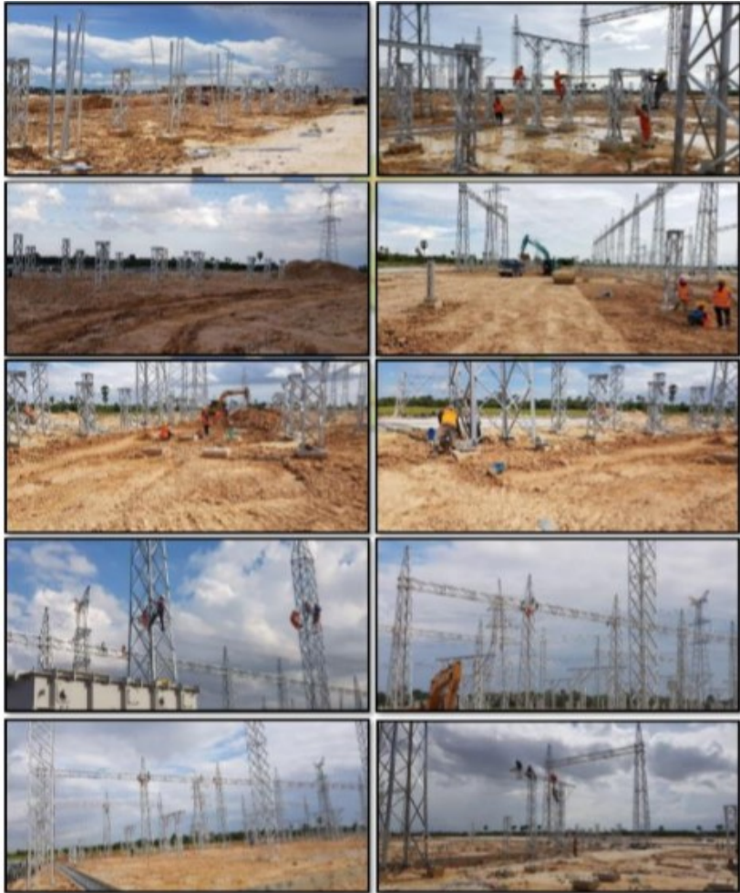
Structure for Substation
