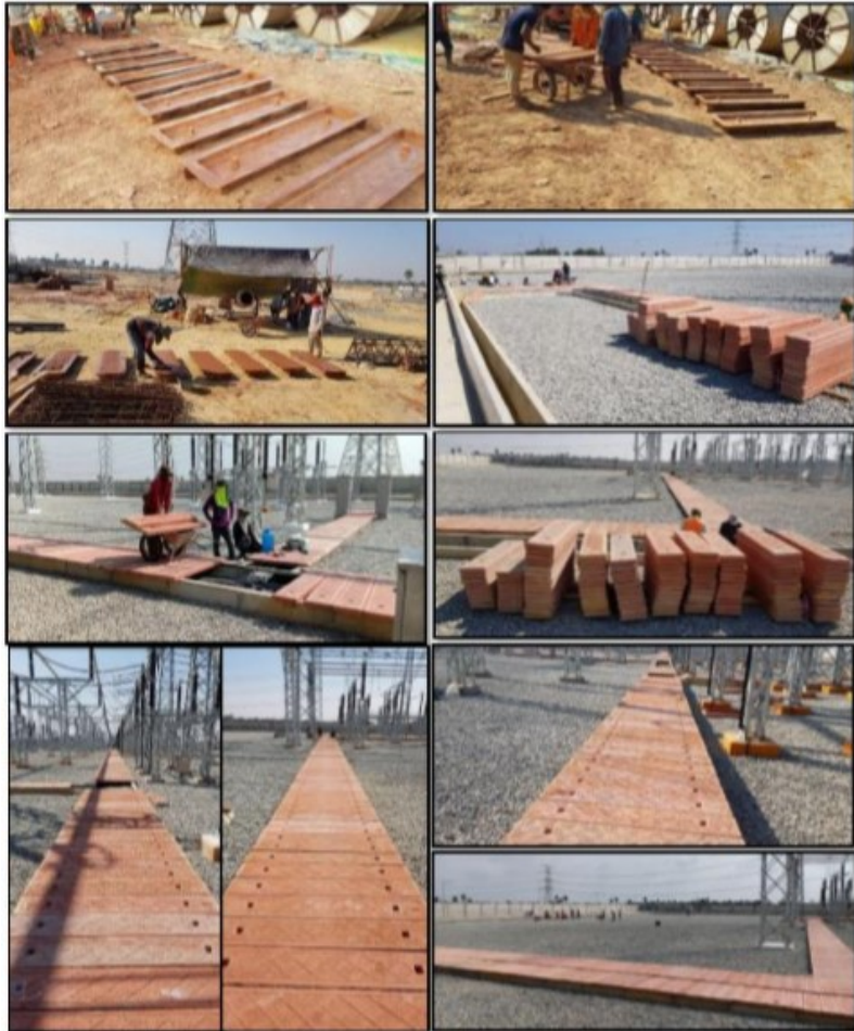
Precast Cover for Cable Trench for Substation
