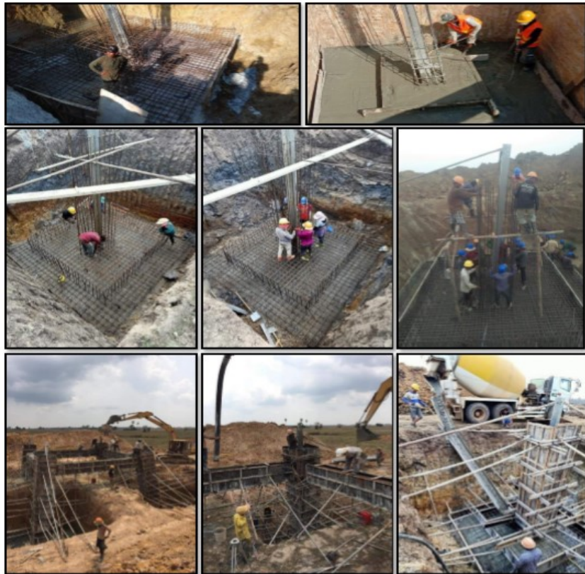
Foundation of Transmission Line
